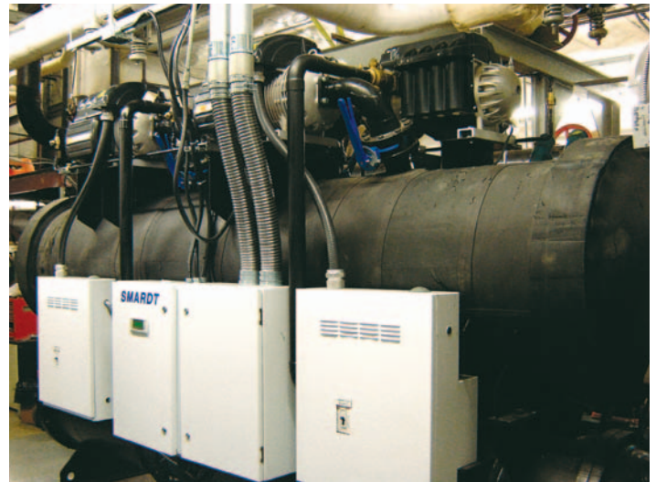
The Smardt 350 tr water cooled chiller installed at the Sears mall at Halifax, Nova Scotia has been delivering reliable energy savings since the day it was commissioned.
